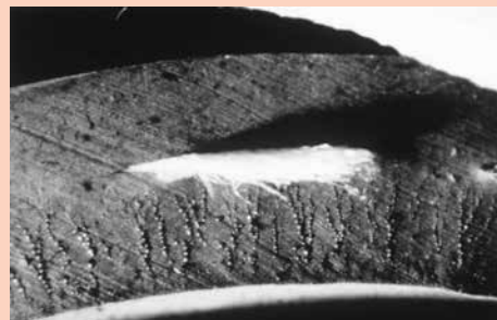
Tube cracking due to electrochemical degradation.
